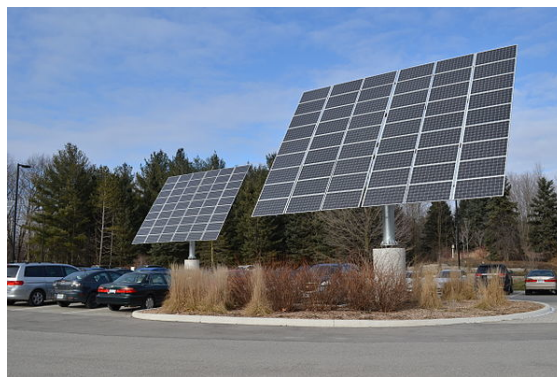
Solar modules mounted on solar trackers
